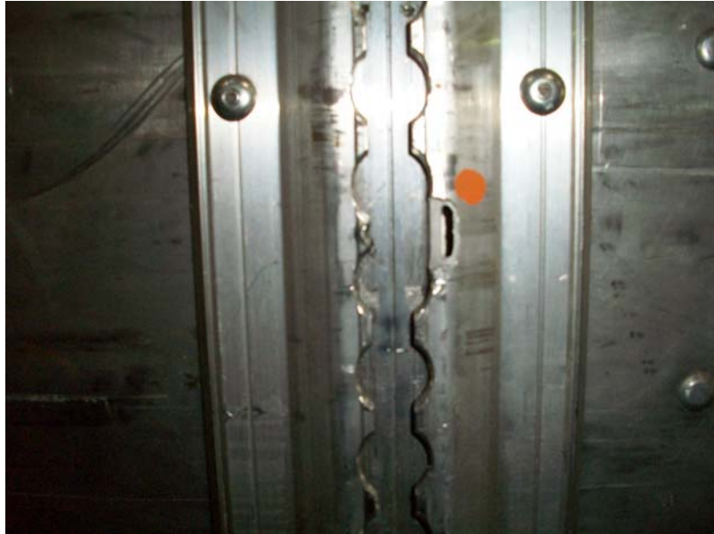
Damaged Track- Missing track lug
