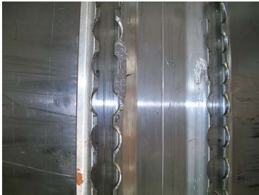
Damaged Track – Surface wear
